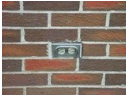
*The weatherproof cover is missing at the patio outlet.
